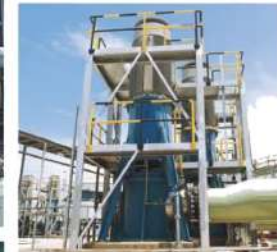
Sea water cooling pumps, Singapore (Size: 800mm, Driver: 790kW)
