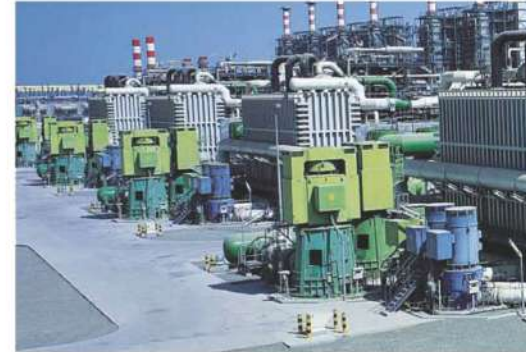
Various seawater pumps in Al Taweela MSF desalination plant, Abu Dhabi, UAE
