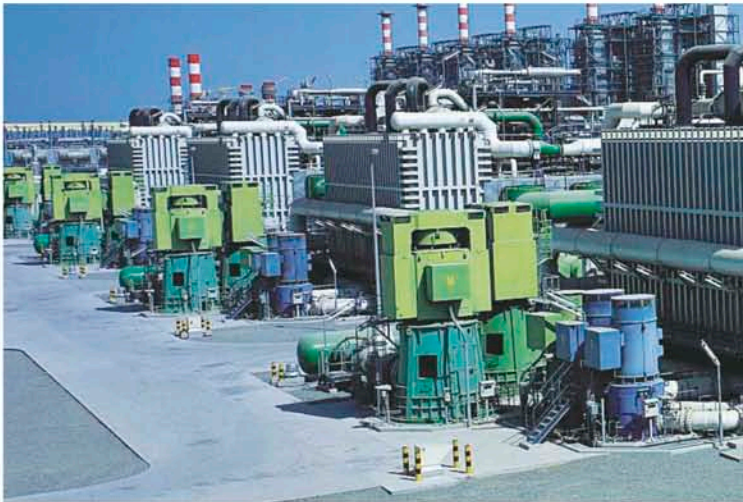
Various seawater pumps in Al Taweela MSF desalination plant, Abu Dhabi, UAE
