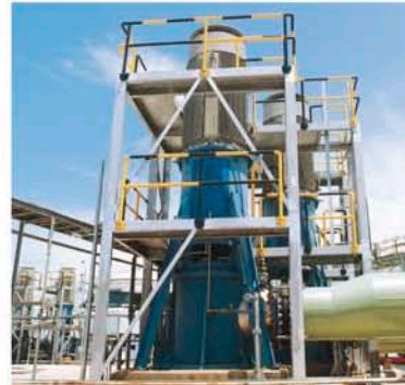
Sea water cooling pumps, Singapore (Size:800mm, Driver:790kW)
